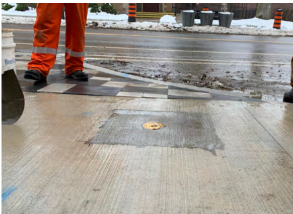
Gas valve box in sidewalk
